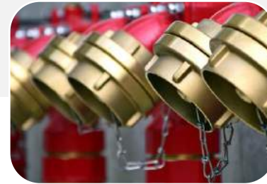
Fire fighting components
